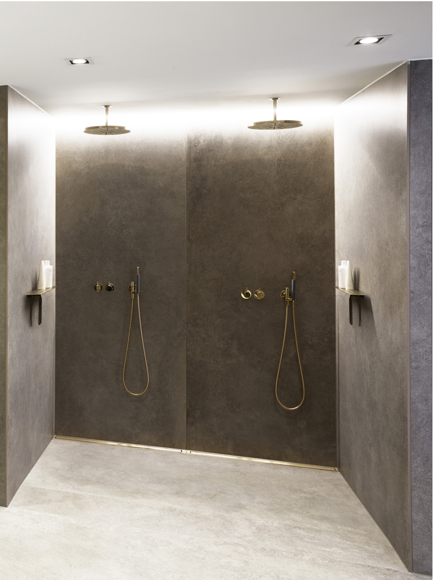
Reframe Collection toilet brush, toilet paper holder, soap shelf and wiper | Brass HighLine Colour bespoke floor drain | Brass
